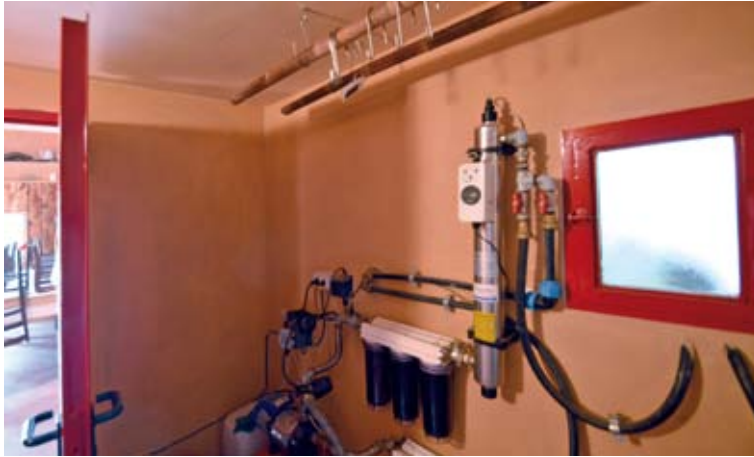
Safe-water making device and inflow pipelines
